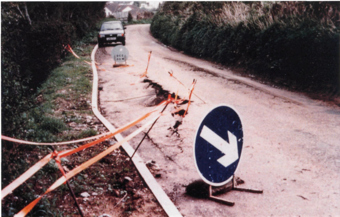
Plate IV Road subsidence caused by badger tunnelling into the road embankment, Devon, England ( C J Wilson, FRCA )
